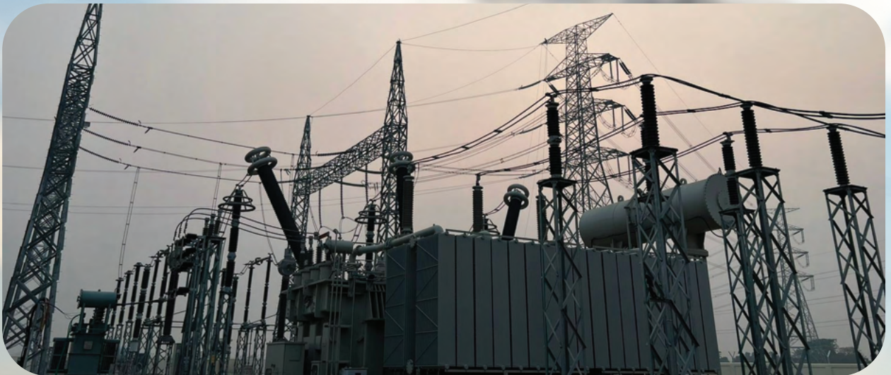
400/132kV, 520 MVA AIS Substation at Rahanpur for Back Feed Power to Adani Power (Jarkhand) India.
