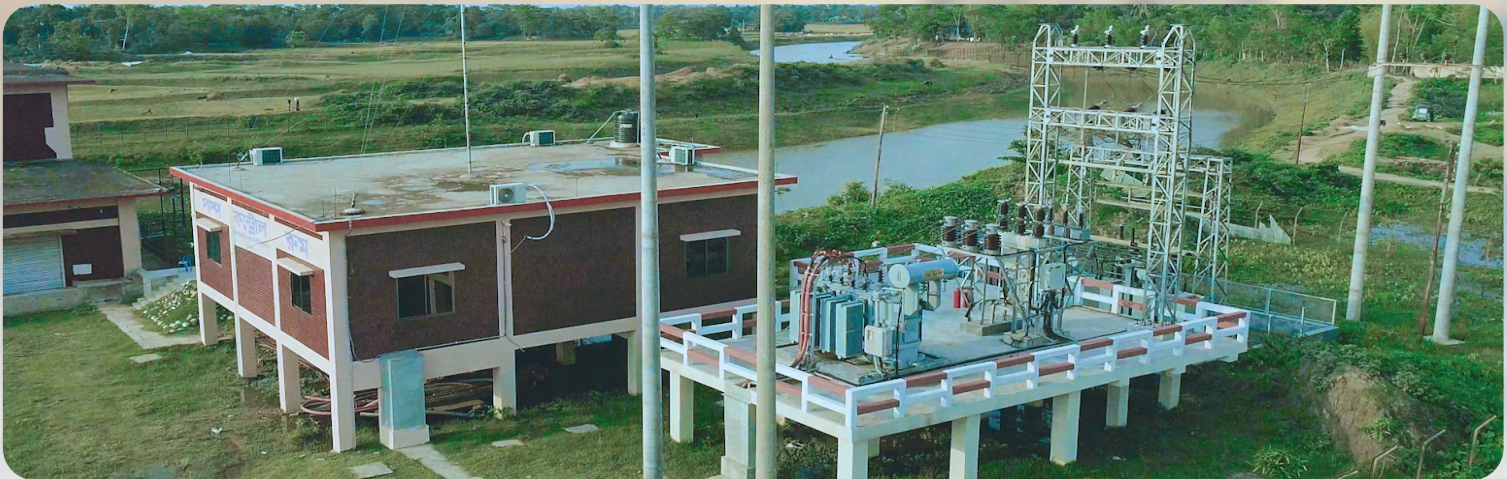
Sigma Engineers Limited (Kashimpur Pump House) Supply, Installation, Testing & Commissioning of 4 MVA, 33/4.2KV Electrical Substation with motor control system and Pump Automation & Additional Works
