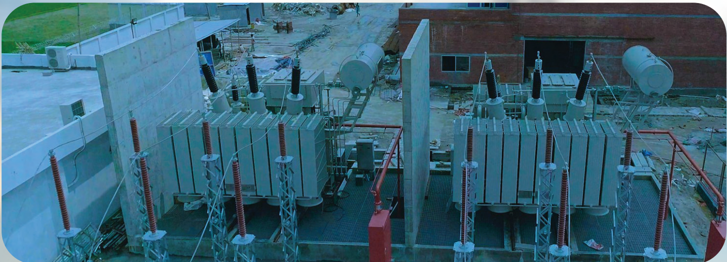
EPC Project: Design, Supply, Installation, Testing & Commissioning of Electrical Balance of plant including 132KV GIS Substation for 163 MW HFO Power Plant Confidence Power Rangpur 113 HFO Power Plant.
