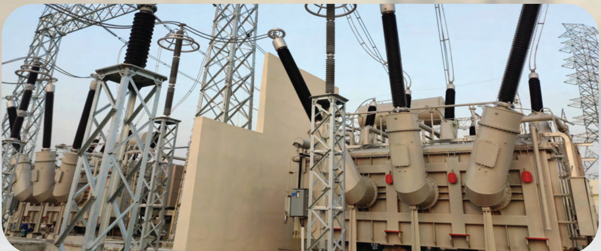
EPC Project: PGCB 400/132/33kV, 250/350 MVA Payra Substation Project at Gopalganj.
