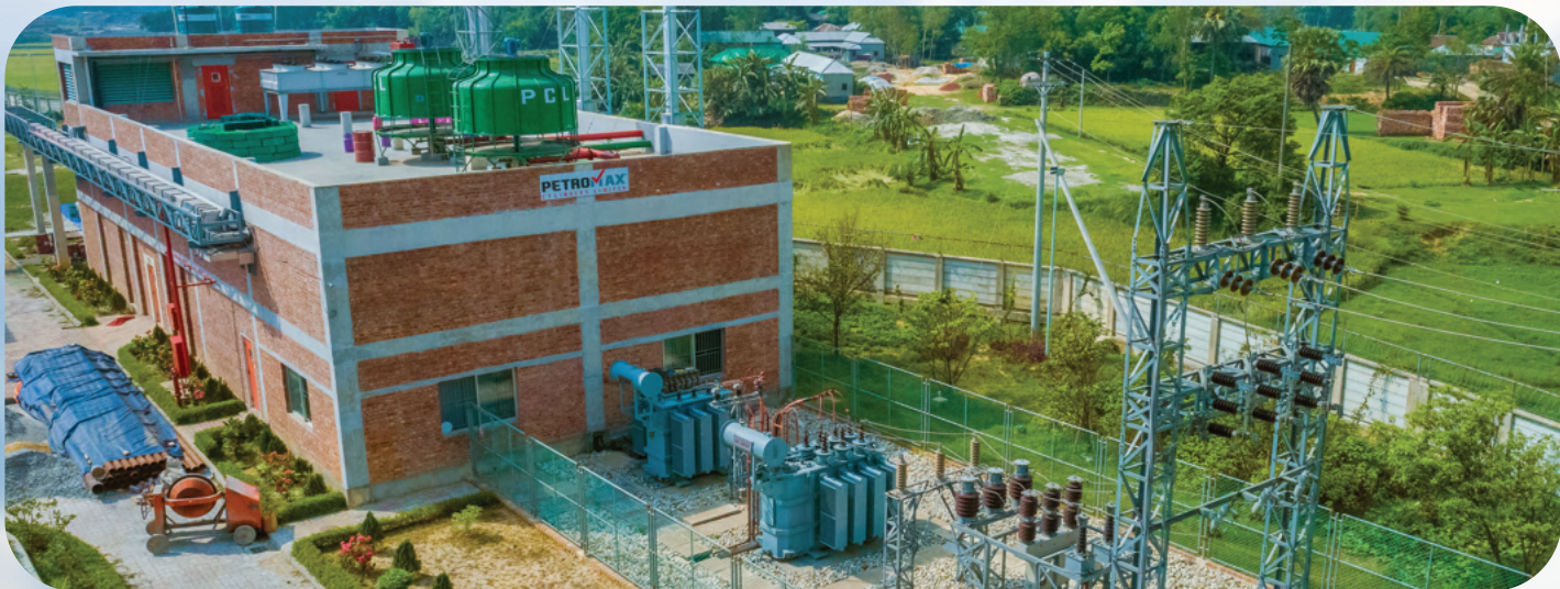
Petromax Cylinders limited: Supply, Installation, Testing & Commissioning of 4 MVA, 33/11kV with 4MVA 11kV/.415kV Electrical Substation with 1000KW GAS Generator Synchronization with REB Including Central Load Monitoring System.
