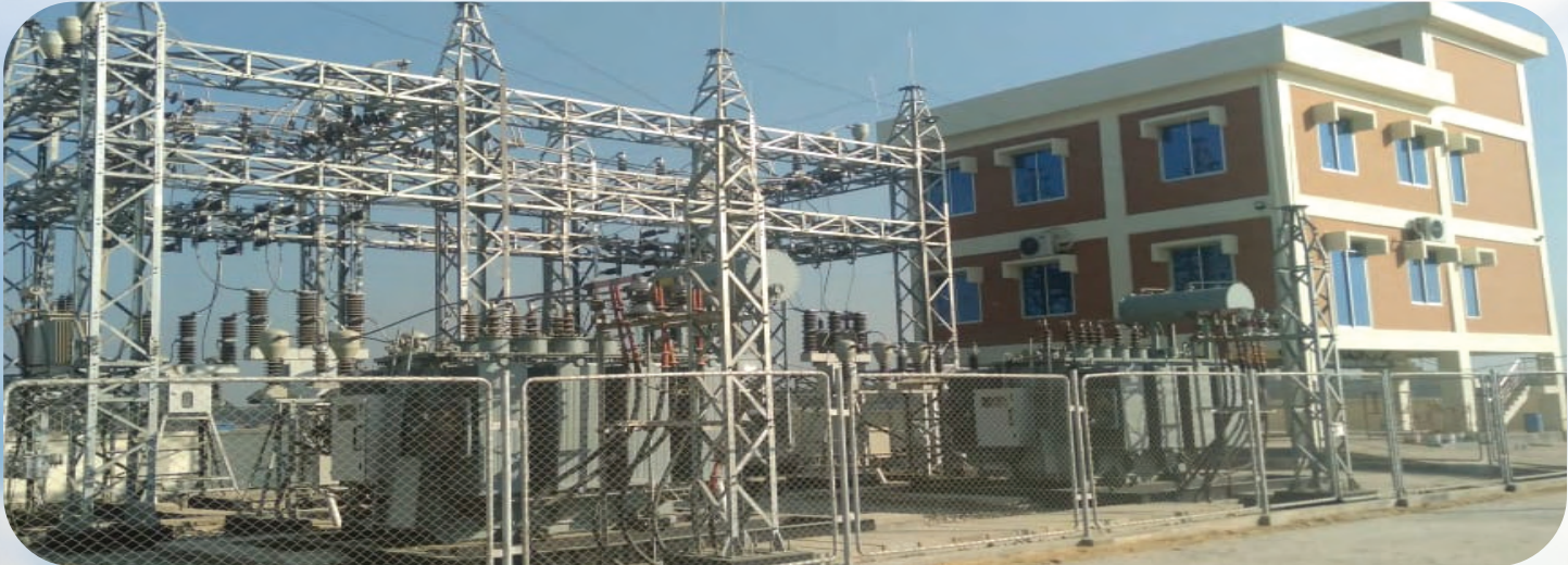
24 Units Turn-Key construction of 10/14 MVA, 33/11Kv Indoor Substation under BREB (Bangladesh Rural Electrification Board) Project at Cox's Bazar, Dhaka, Mymensingh, Chittagong, Sylhet, Rajshahi, Rangpur, Khulna, and Barisal.
