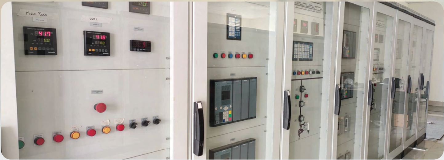
EPC Project: 400KV Control, Relay and Protection Panel at PGCB 400kv Payra Substation (Gopalganj)
