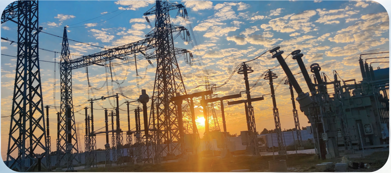
Design, Supply, Installation, Testing and Commissioning of 400 kV outdoor GIS Substation at Bogura (west) & Rahanpur and Upgradation/Extension of Gopalganj and Chapainawabganj (old) Substation on turnkey basis, ADB
