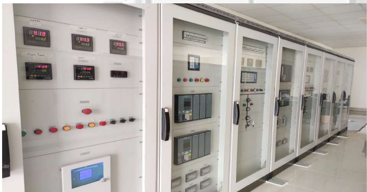
Control & Protection System Gopalgong HV Substation
