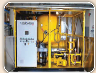
Transformer Oil Centrifuging Machine
