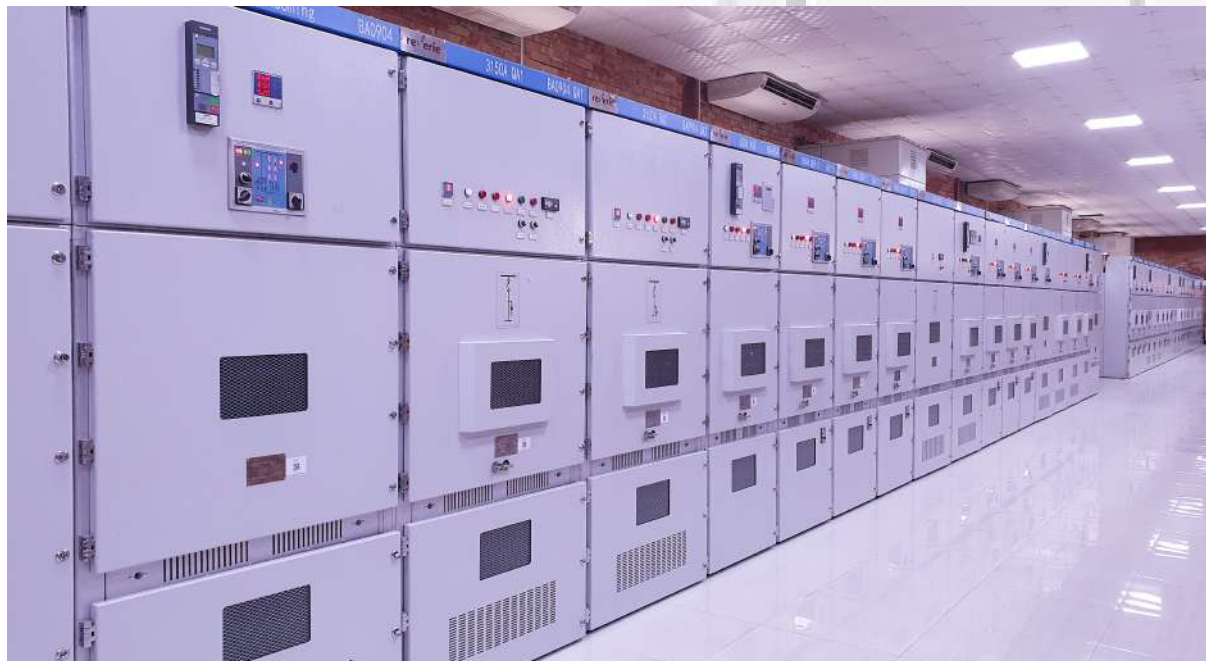
Control & Protection System Desh Energy Chandpur
